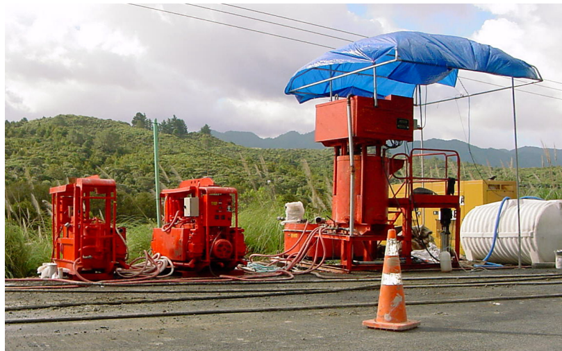
Figure 6. Grout Mixing Plant
