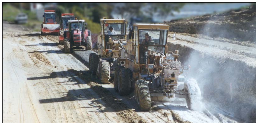
Photo 1: Subgrade stabilising - Tandem hoers, particle sizer, padfoot roller and smooth drum roller.
