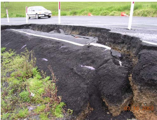
Figure 1: A recent New Zealand road underslip
