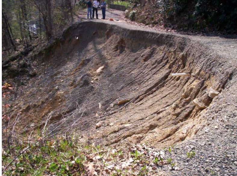
Figure 10. Failure caused by water service leak.
